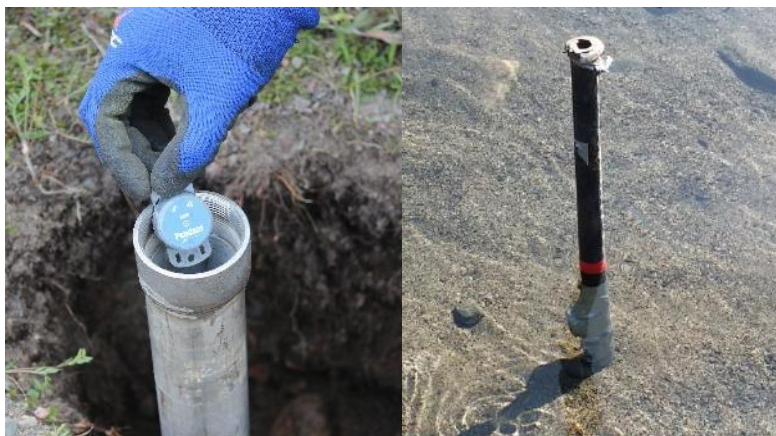
Figure 12 - Temperature sensors inside the pipe for measuring ground temperature (left) and attached to the pipe for measuring the temperature inside and below the river (right)
